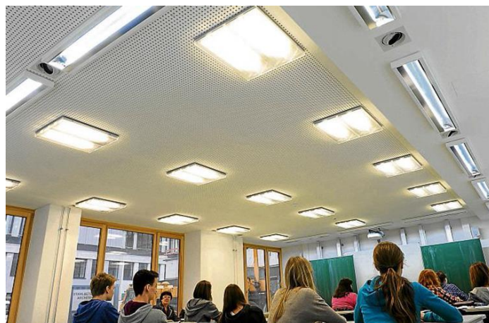
Figure 7 – Miesbacher Merkur (2013). HCL design in a classroom (FL-Technology, Bavaria).
